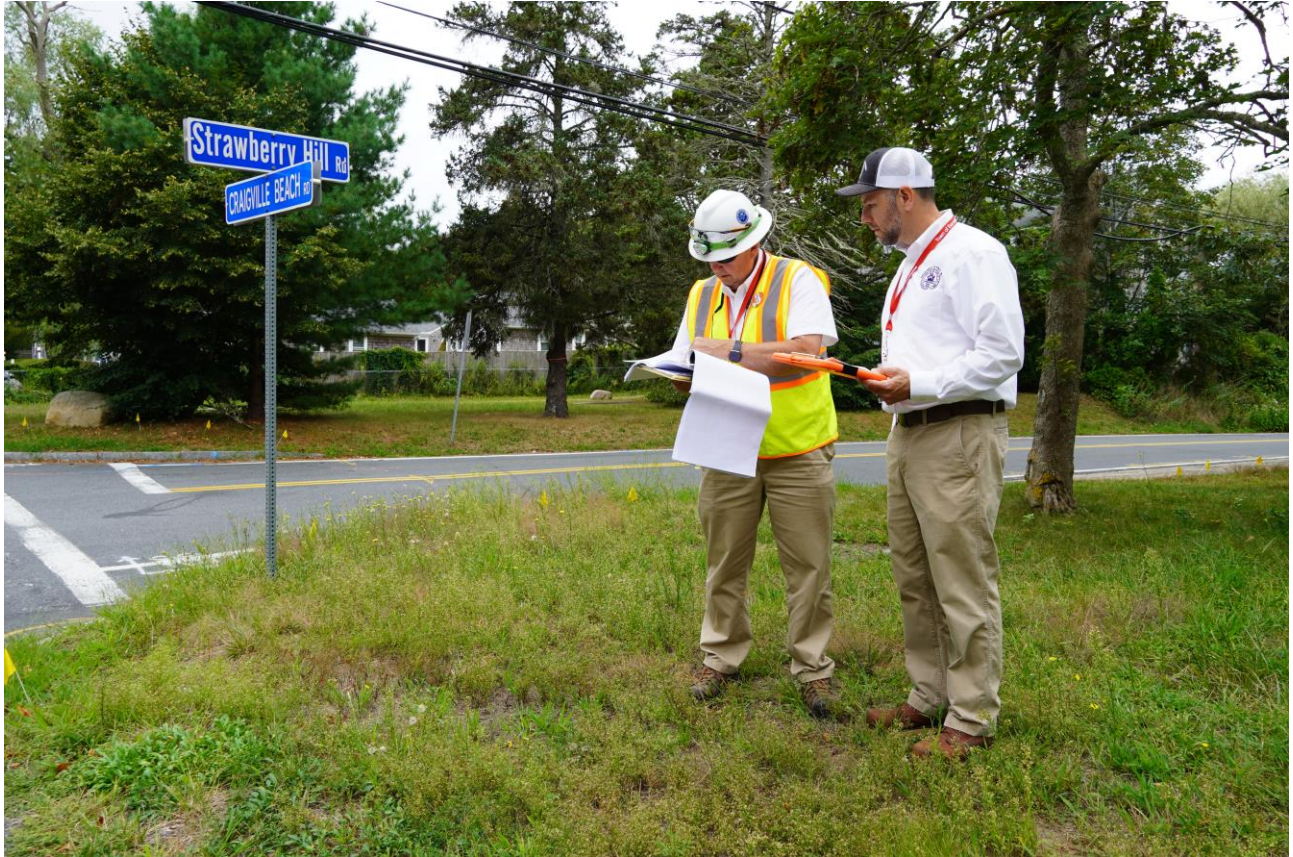
Pictured above Construction Inspector Stephen Porter and Senior Project Manager Paul Ruzala, P.E. who are working on the Strawberry Hill Road Sewer Extension project.
