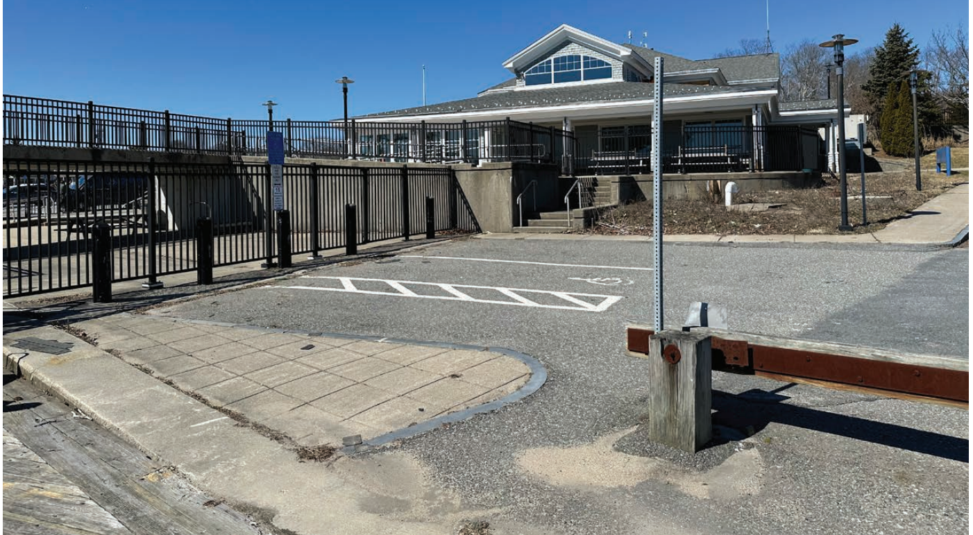
Figure 29: Closed Public Access under Steamship Authority Terminal, looking north Source: BRR, 2024
