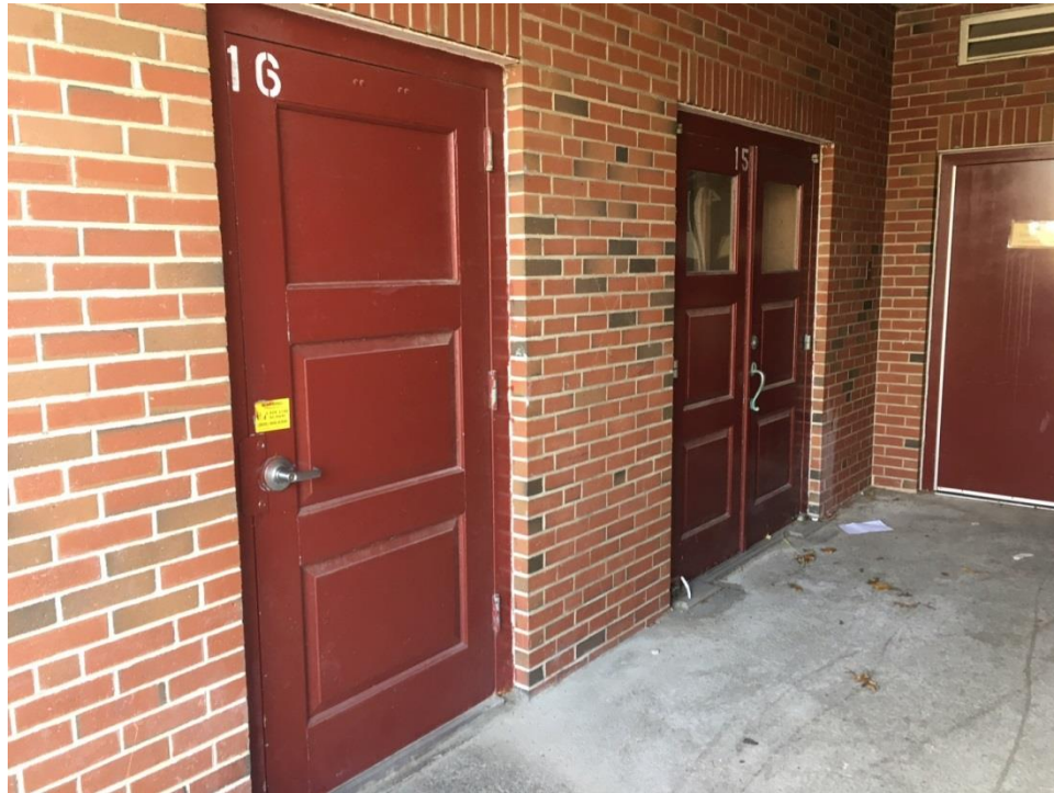
Hyannis West Door Needing Replacement
