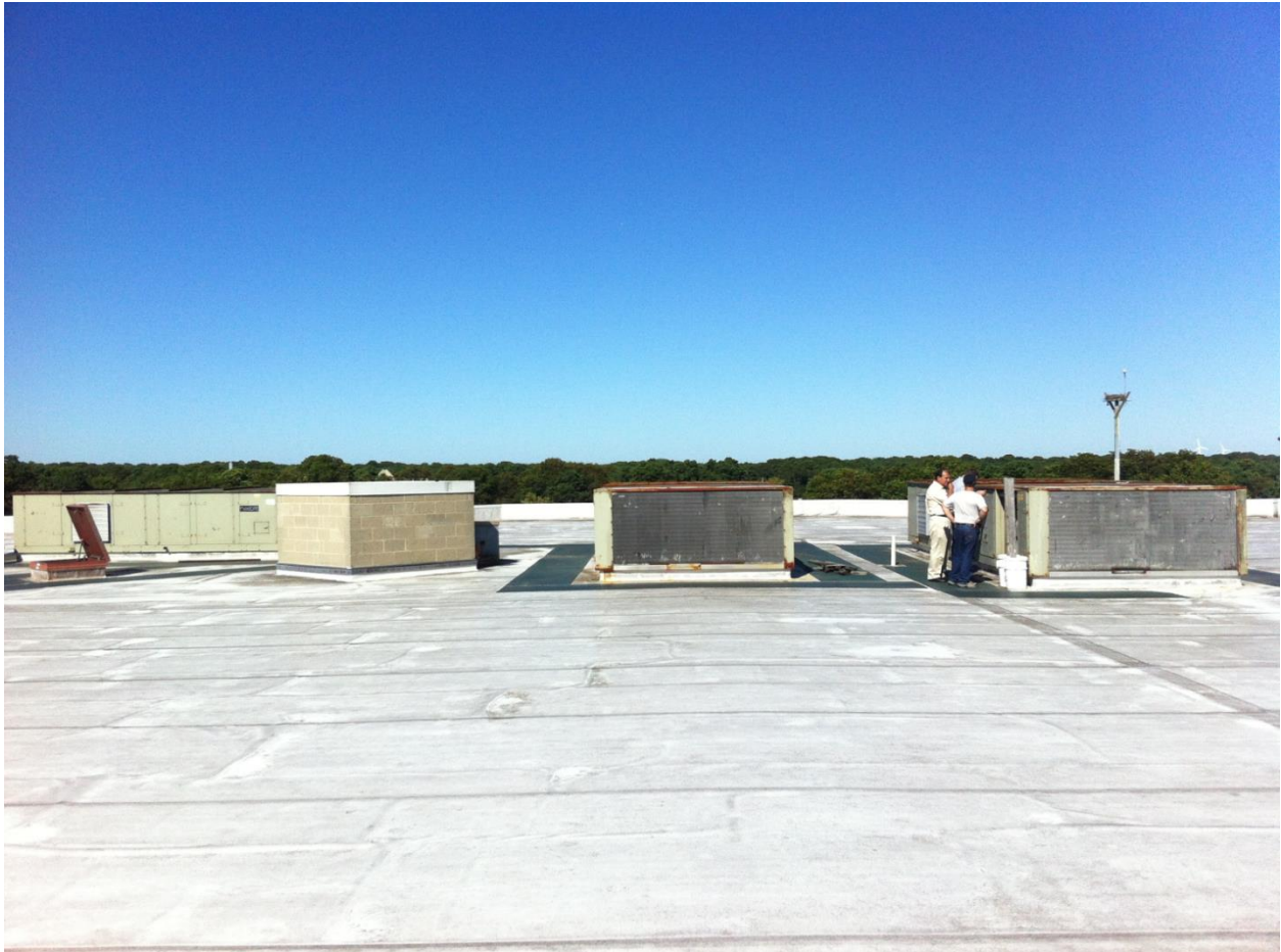
Roof Top Unit Ventilators (RTU)
