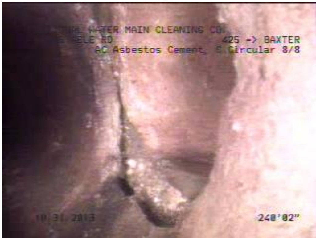
Barnstable Road Deteriorating Pipe
