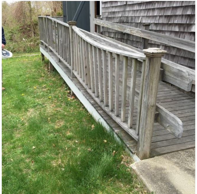
Old Jail House Interior and Exterior Repairs Needed
