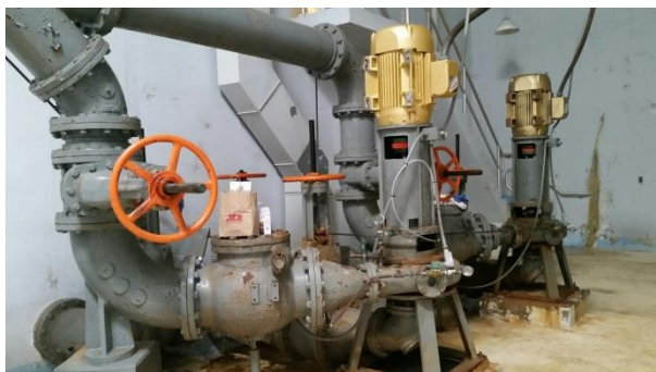
Freezer Road Pumps
