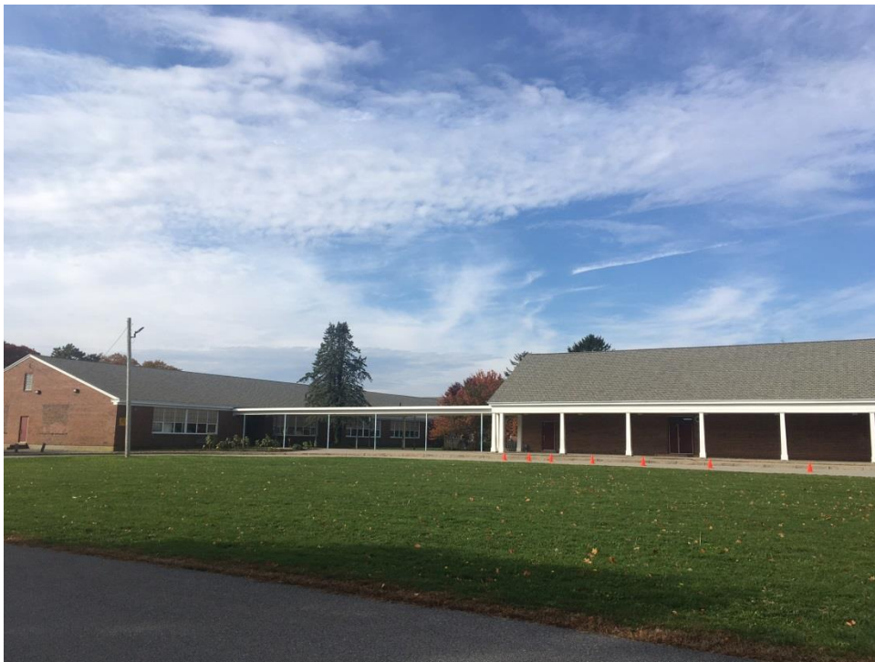
Hyannis West Elementary School Needs Roof Replacement
