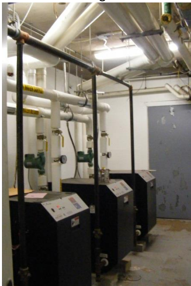
Mechanical Controls to Cooling System
