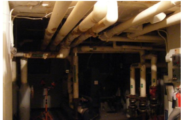
Mechanical Induct system
