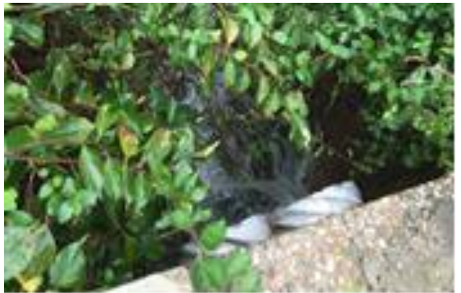
Storm Water Drainage
