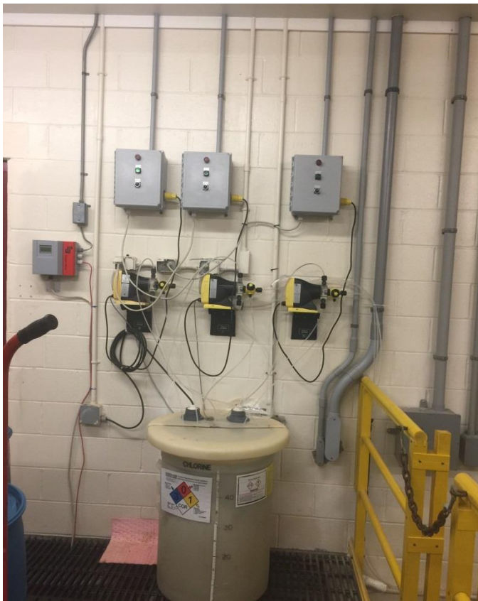
Water System Components: Pumps and Electrical
