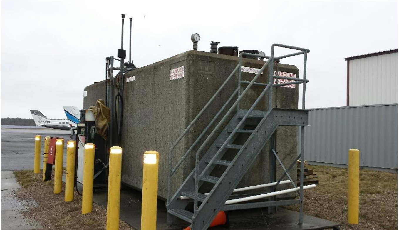
Mo-Gas and Diesel Fuel Con-Vault
