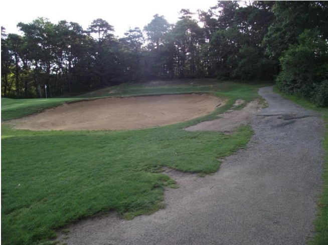
Hole #13 Deteriorating Cart Path & Bunker
