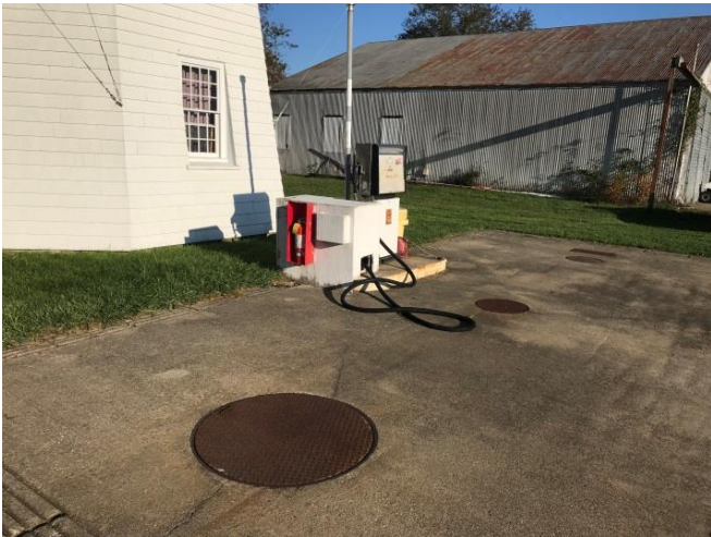
Cape Cod Air Field Fuel Tank Pump
