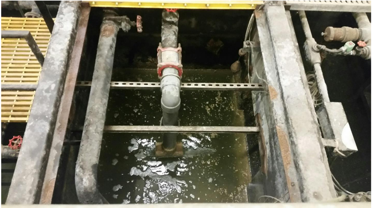
Denitrification Sand Filter
