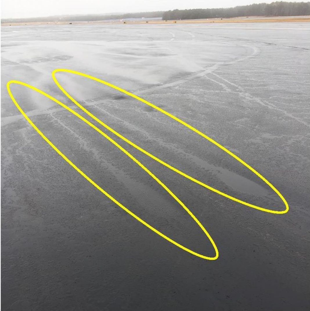
Pavement depressions due to heavy aircrafts
