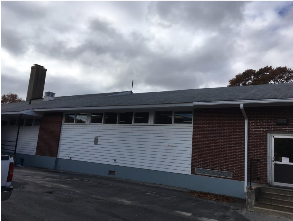
Centerville Elementary School Needs Roof Replacement
