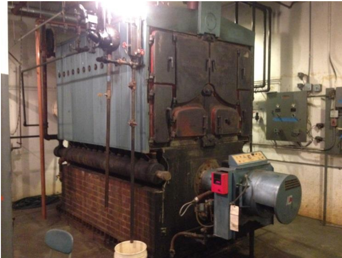
Cotuit Elementary School Boiler
