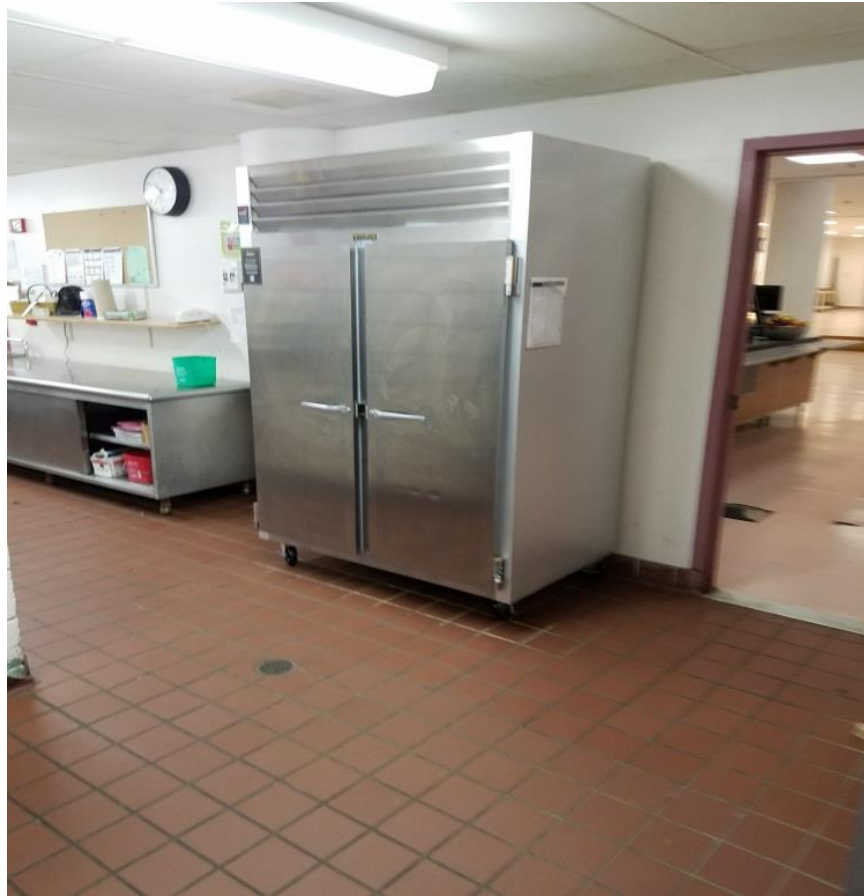
Barnstable Intermediate School Reach-In Freezer
