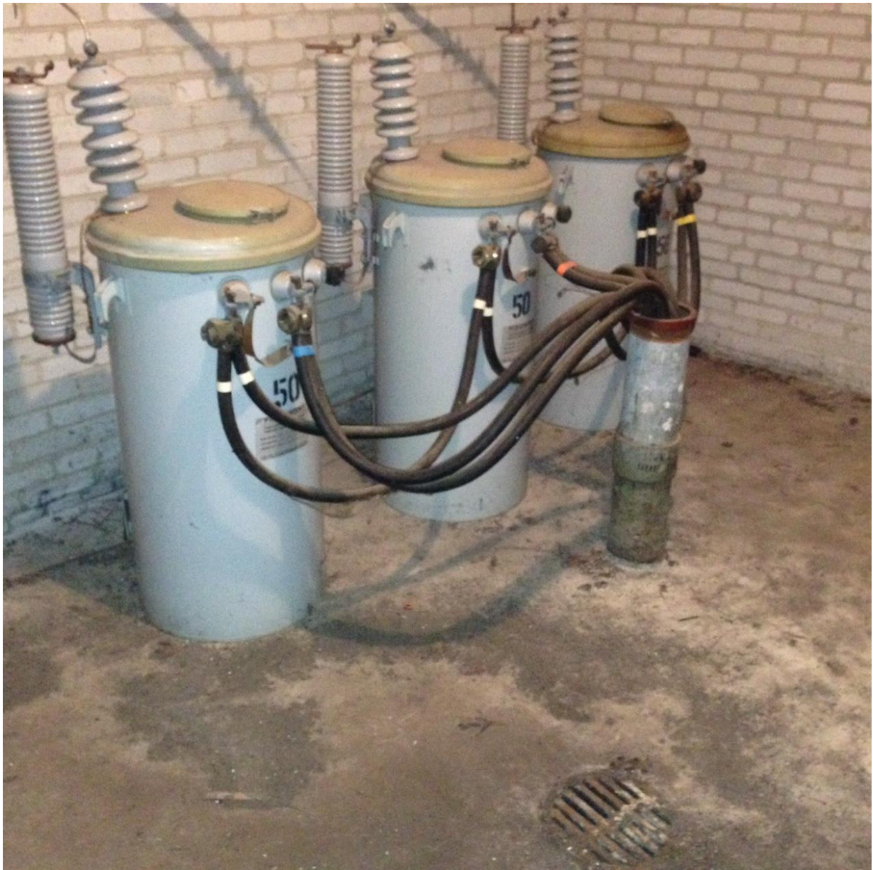
Typical Underground Transformer Vault
