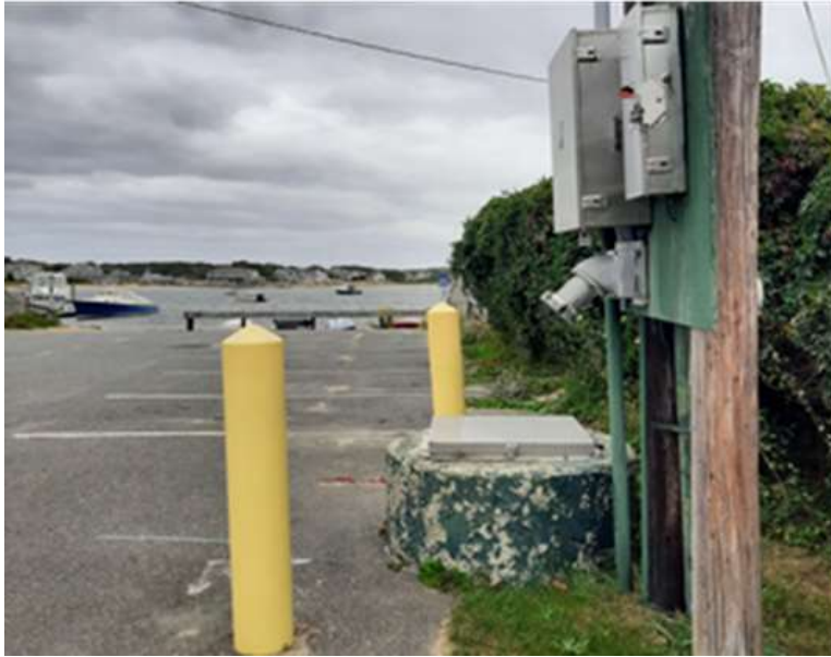
Photo 2: Bayshore Road Pump Station
