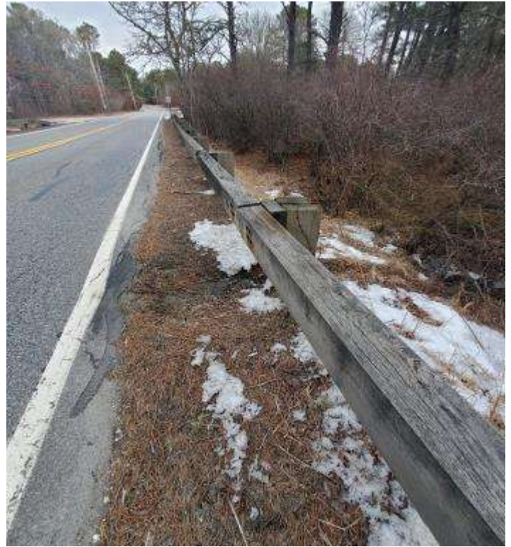
Runoff from Santuit Newtown Road under the guardrail to Lovells Pond. Taken February 2021.
