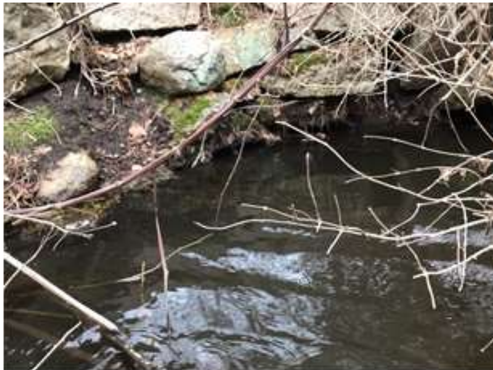
Photo 2: Looking at completely submerged culvert on downstream side of Rosa Lane.
