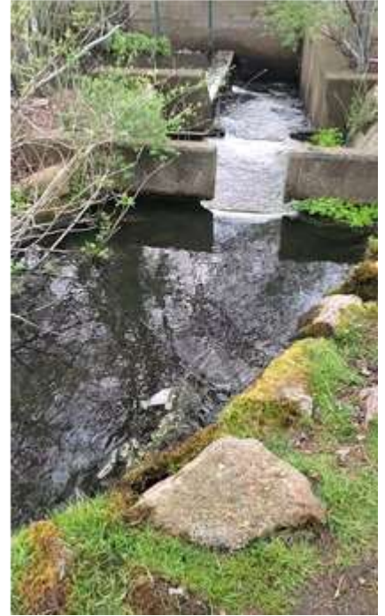
Worn steps and pools along fish ladder.
