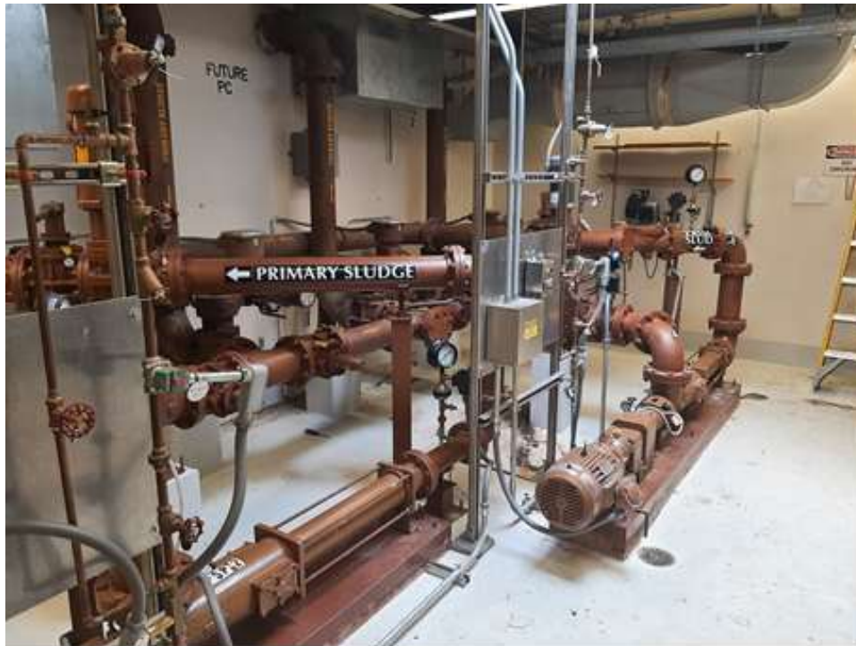
Primary Pump Room
