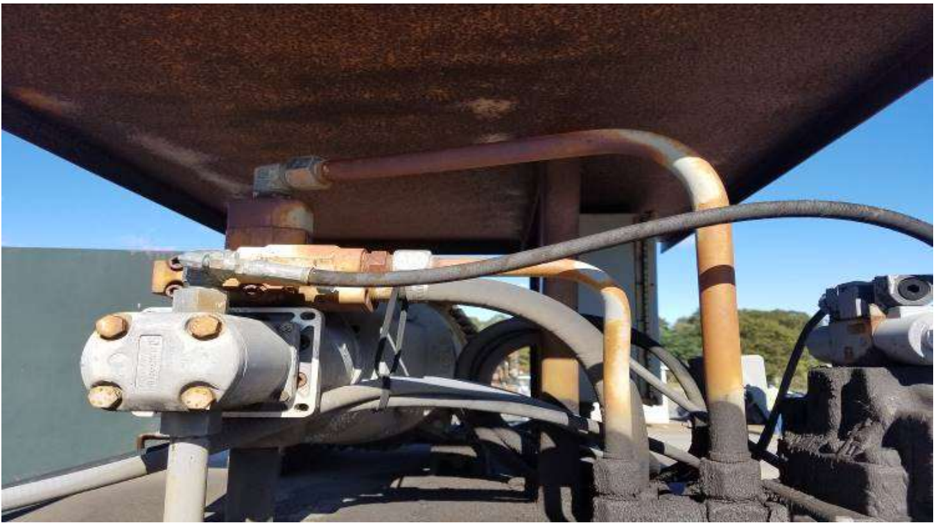
Compactor Units at Transfer Station
