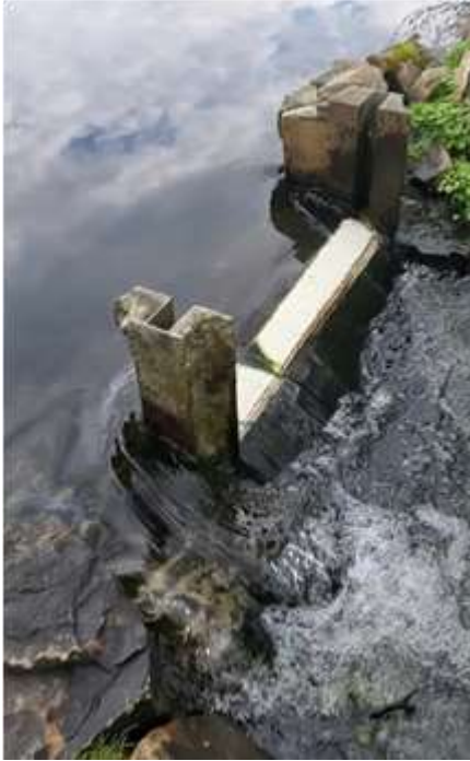
Stone damage and missing stones around the water control structure. Taken on 4/28/2021
