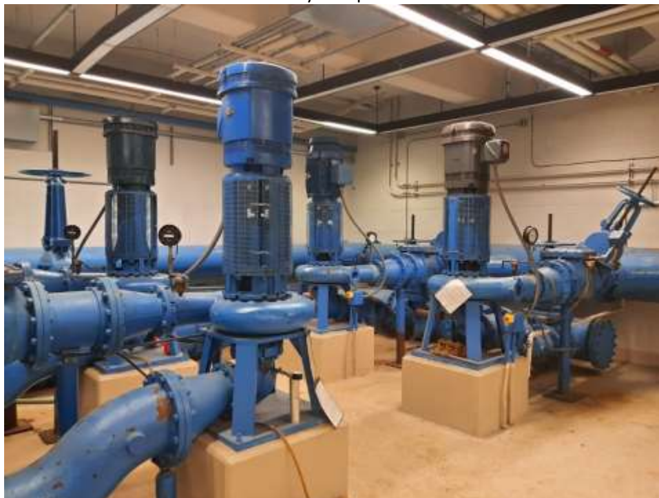
WPCD Effluent Pumps, installed in 1980
