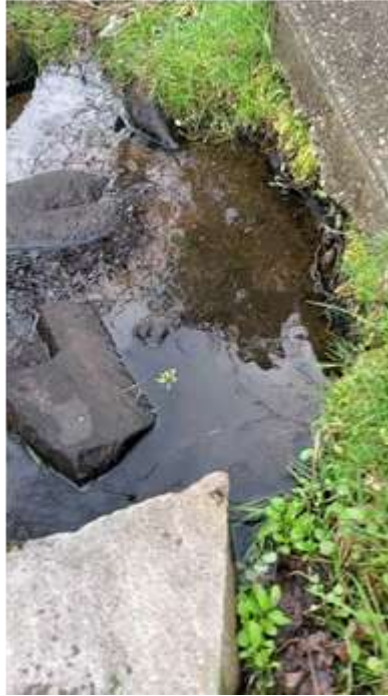
Water flow from pond under the sidewalk caused undermining. Taken on 4/28/2021
