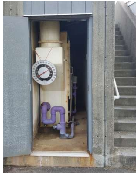
Photo 2: Odor Control System Access
