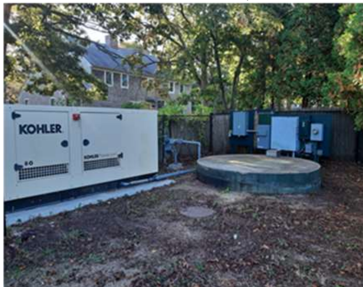
Photo 4: Marks Path Pump Station
