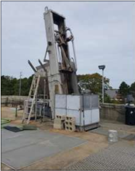
Photo 1: Mechanical Bar Screen
