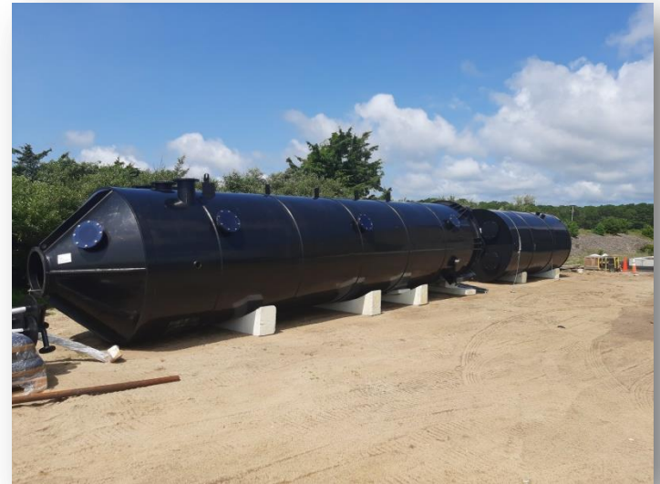
Odor Control Systems, WPCF
